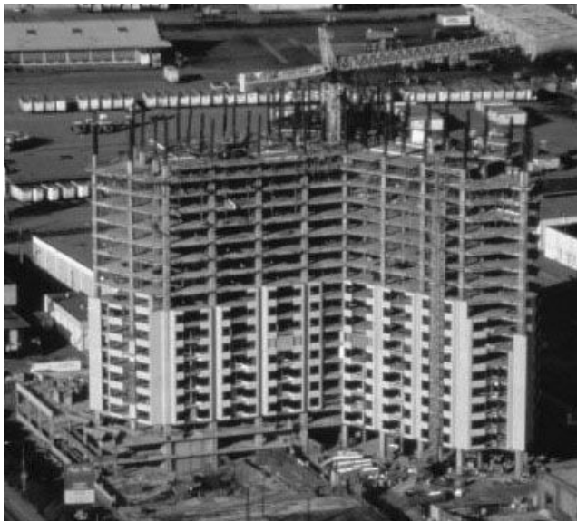
PHOTO 4.1 A 30-story reinforced concrete building under construction. The Pacific Park Plaza is one of the largest reinforced concrete structures in the San Francisco Bay area. It survived the October 17, 1989, Loma Prieta earthquake without damage. Instrumentation in the building recorded peak horizontal accelerations of 0.22g at the base and 0.39g at the top of the building (courtesy of Mr. James Tai, T.Y. International, San Francisco).
