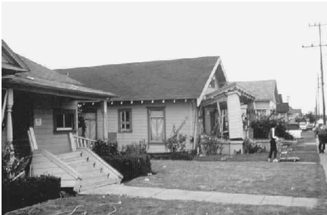
FIGURE 7.5 Houses damaged due to cripple wall failure, 1983 Coalinga Earthquake (courtesy of EQE International).
