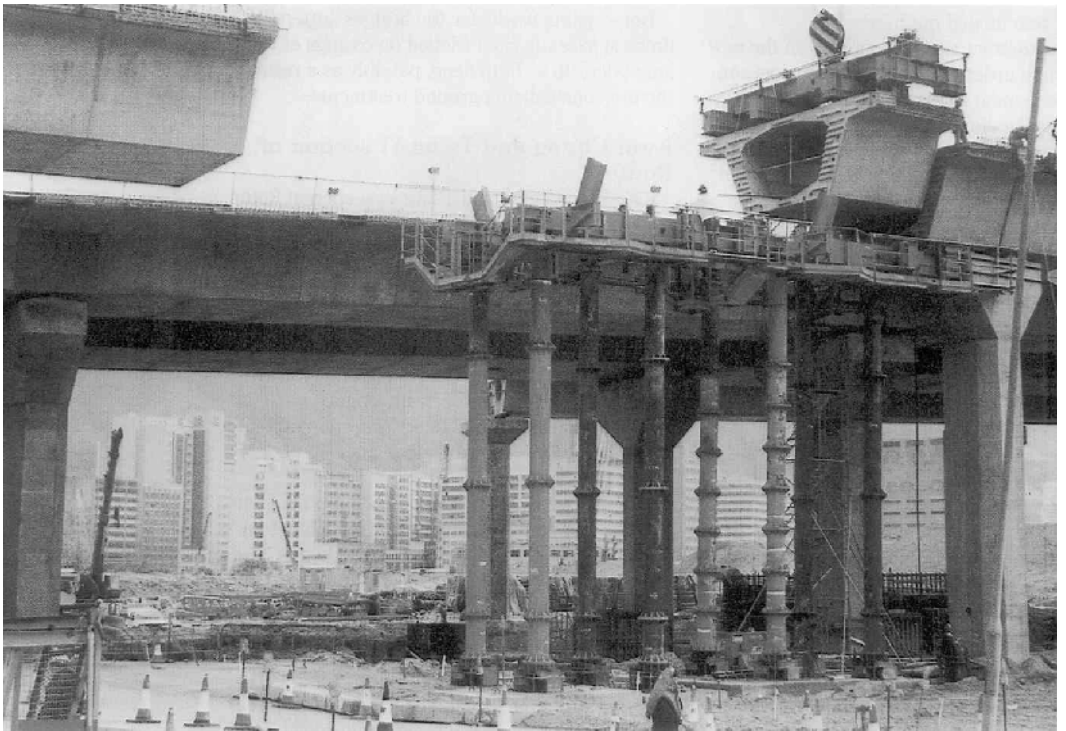
PHOTO 5.8 West Kowloon Expressway Viaduct, Hong Kong, during construction, comprising 4.2 km dual three-lane causeway connecting Western Harbor Crossing to new airport (courtesy Institution of Civil Engineers, London, and [5]).
